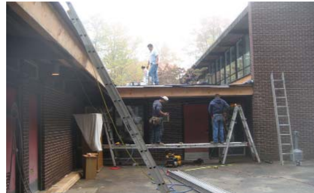
Workers installing a new church roof at Holy Communion, Mahopac at a cost of approximately $32,000.
